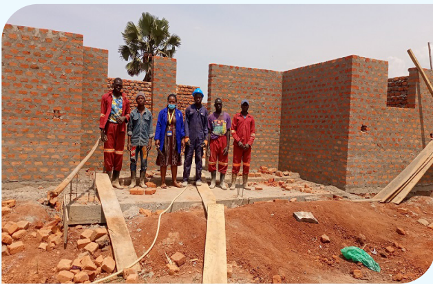
NCBC Trainees constructing a residential house in ROM village Karo sub county –Gulu District under the supervision of Mwaka Construction Company Limited.
